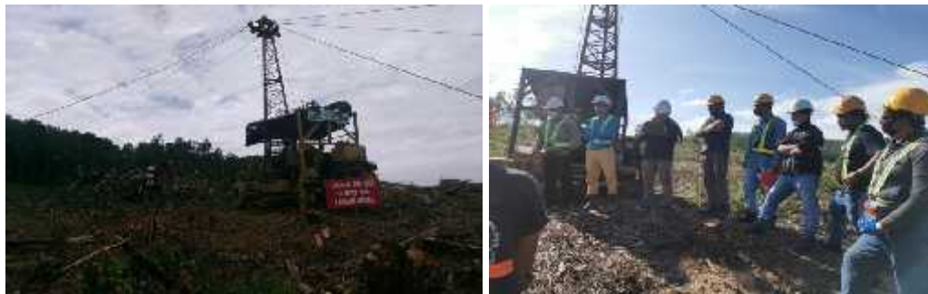
Cable Yarder System
